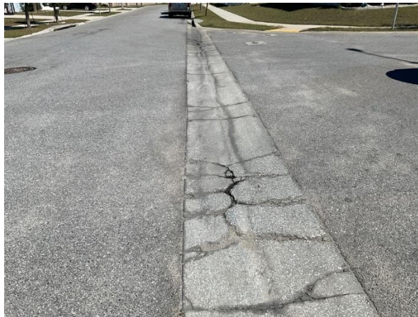
Concrete cracks at Taft Drive and Jefferson Street intersection
