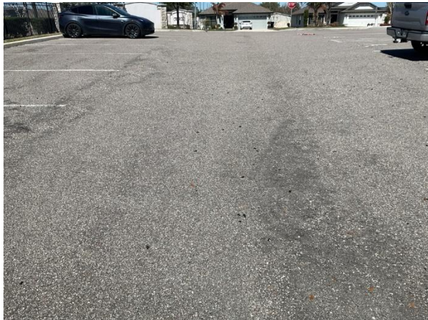
Pavement overview at Citrus Point pool with pavement deterioration evident
