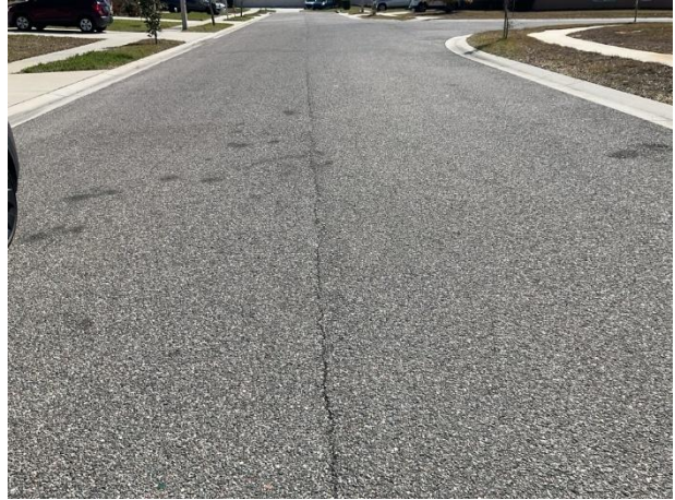
Pavement cracks at Buchanan Drive
