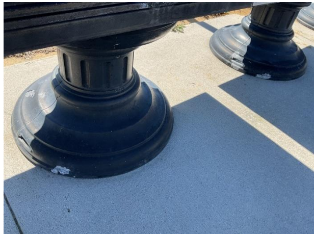
Mailbox station finish deterioration
