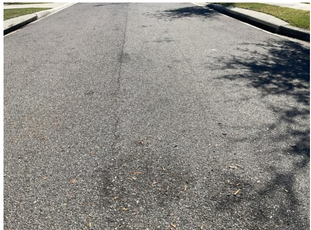
Pavement cracks and deterioration at Buchanan Drive
