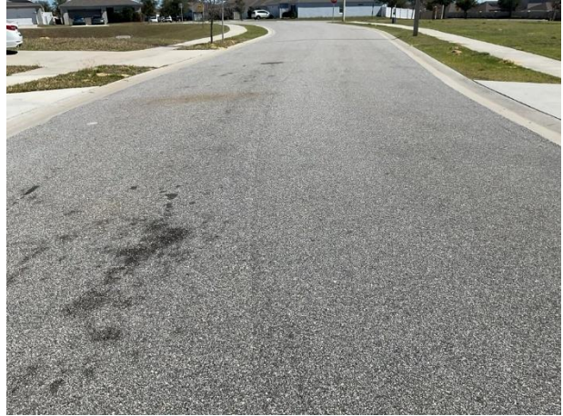
Pavement overview at Taft Drive with vehicle fluid stains evident
