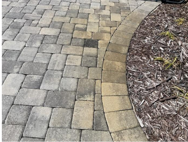
Stains at pavers
