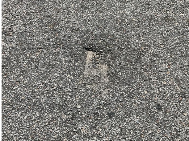
Pavement deterioration at Taft Drive
