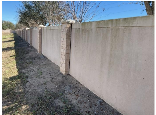
Concrete perimeter wall overview with organic growth evident
