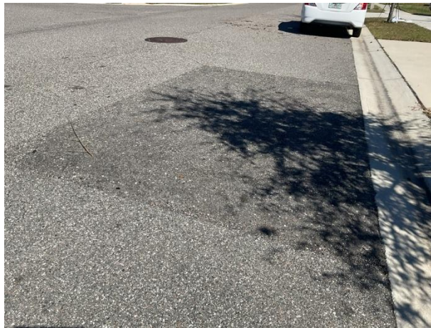
Previous repairs evident
