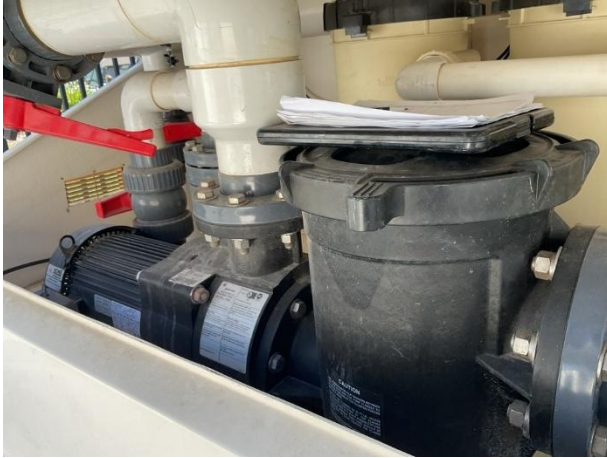
Pool mechanical equipment
