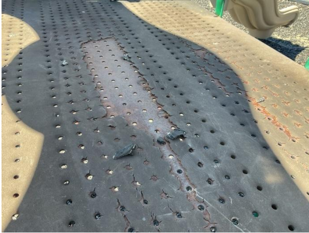
Equipment finish deterioration and rust at citrus point pool
