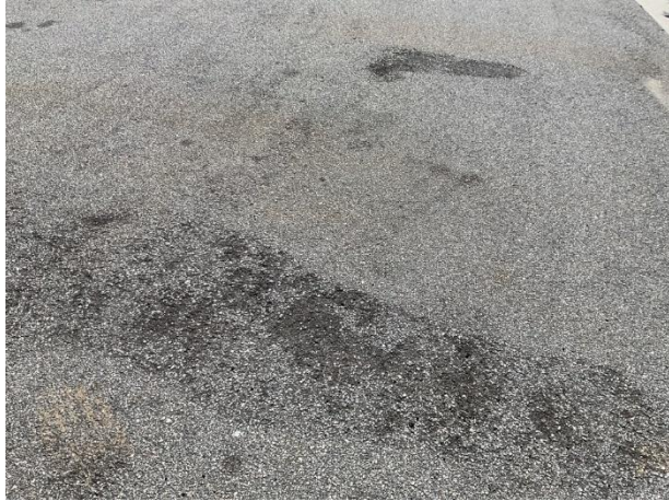
Pavement deterioration at Fillmore Court
