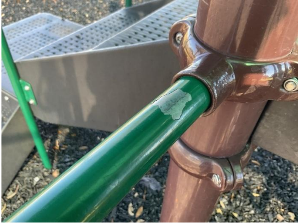
Equipment finish deterioration at Citrus Isle
