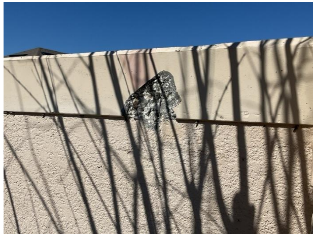
Wall concrete spalls at North Ridge Estates entrance perimeter
