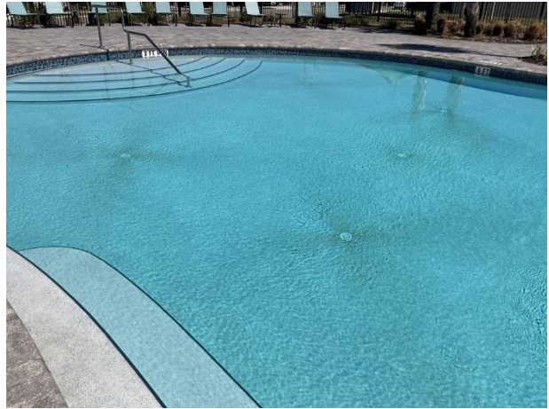
Pool plaster overview with plaster discoloration evident
