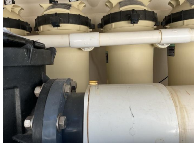
Pool pumps and filters
